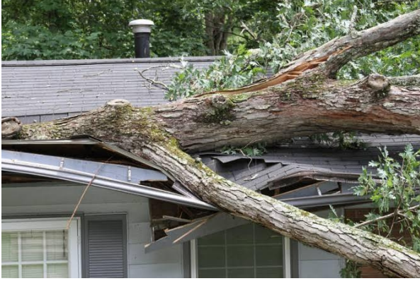
Figure 4 Tree storm damage
