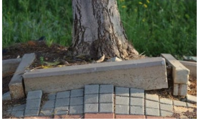
Figure 5 Pavement damage due to tree roots
